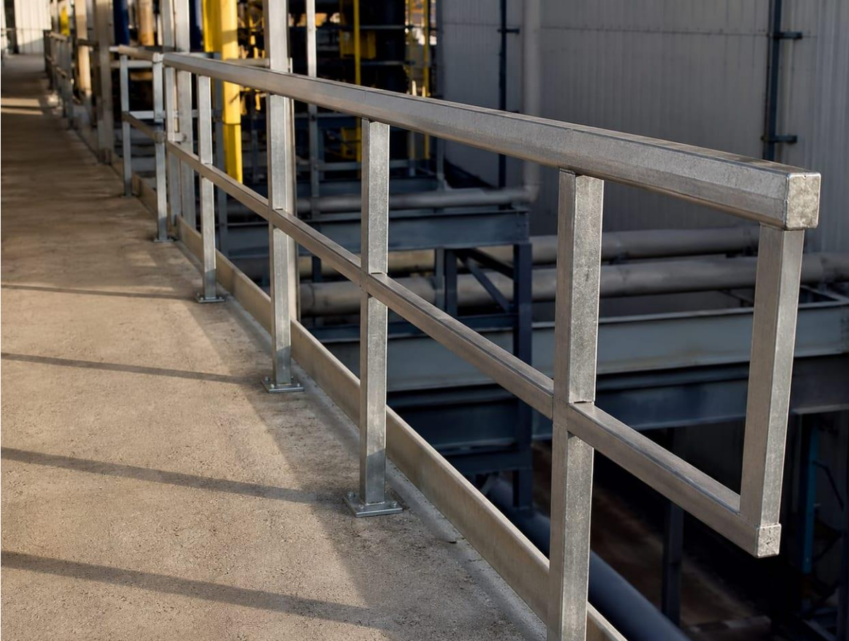
Galvanized square-section handrail on base plates along a walkway.
