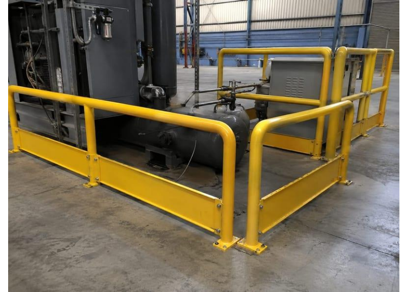
Tubular guard rail around process equipment.
