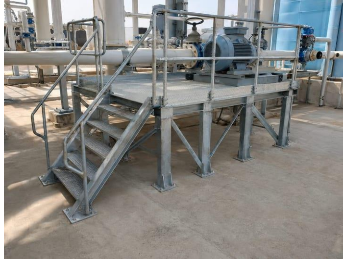
Galvanized platform with stair and handrails serving a motor and pump set.
